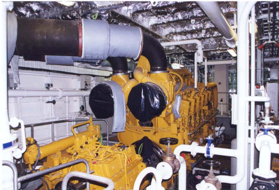
Figure 3 Main Machinery Room
